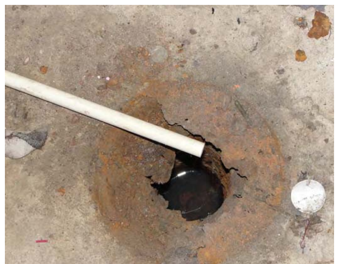
Structural Deficiencies – Unsafe and Unsanitary Conditions
