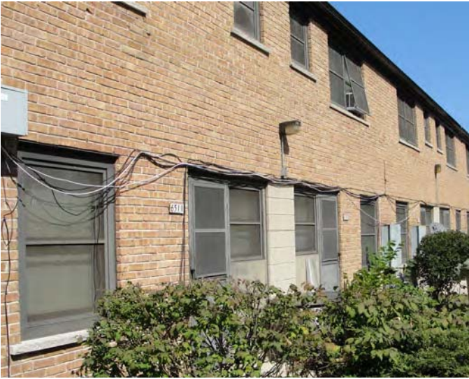
Structural Deficiencies – Window AC Units & Service Retrofits
