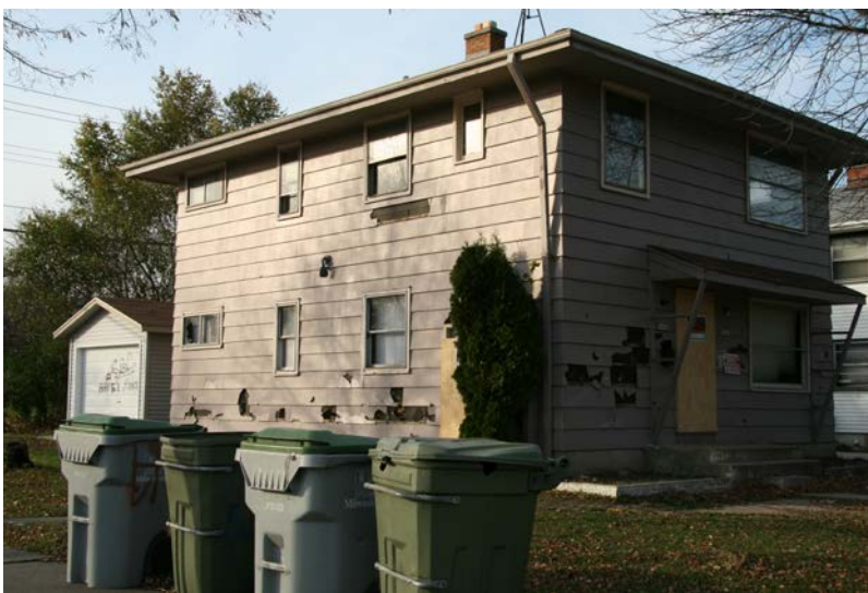
Boarded up home in with holes/missing siding (5641-5643 N. 61 st St.).
